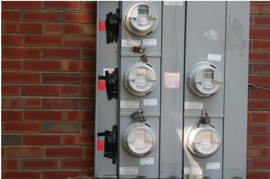
Unit 30: Taped breakers; possibility of not tripping when necessary
