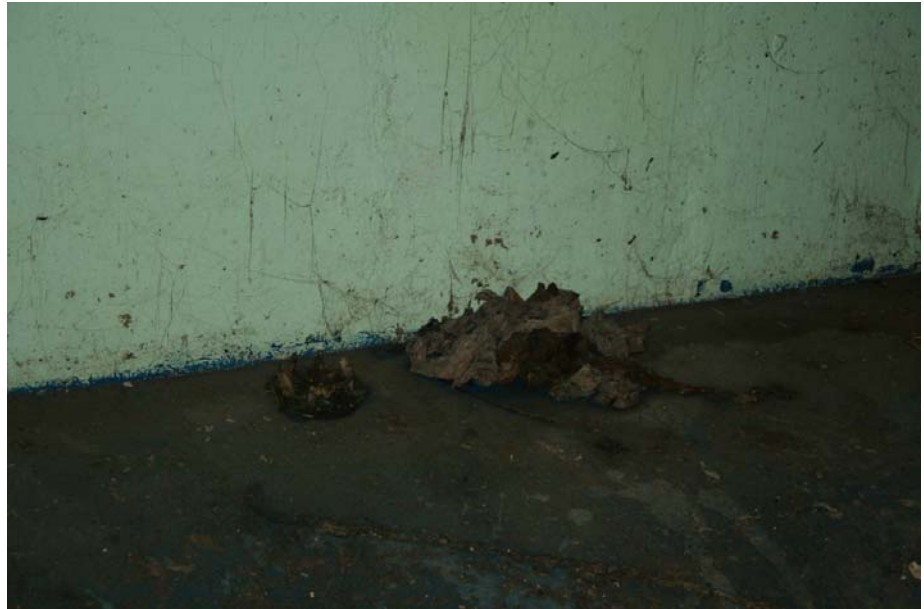
Unit 70: Dried paper and feces from sewage leak
