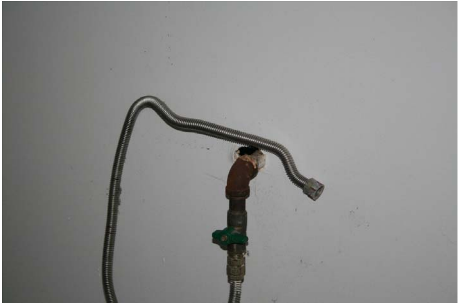
Unit 10: Uncapped gas line
