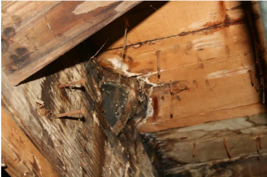
Unit 75: Active water leak from toilet
