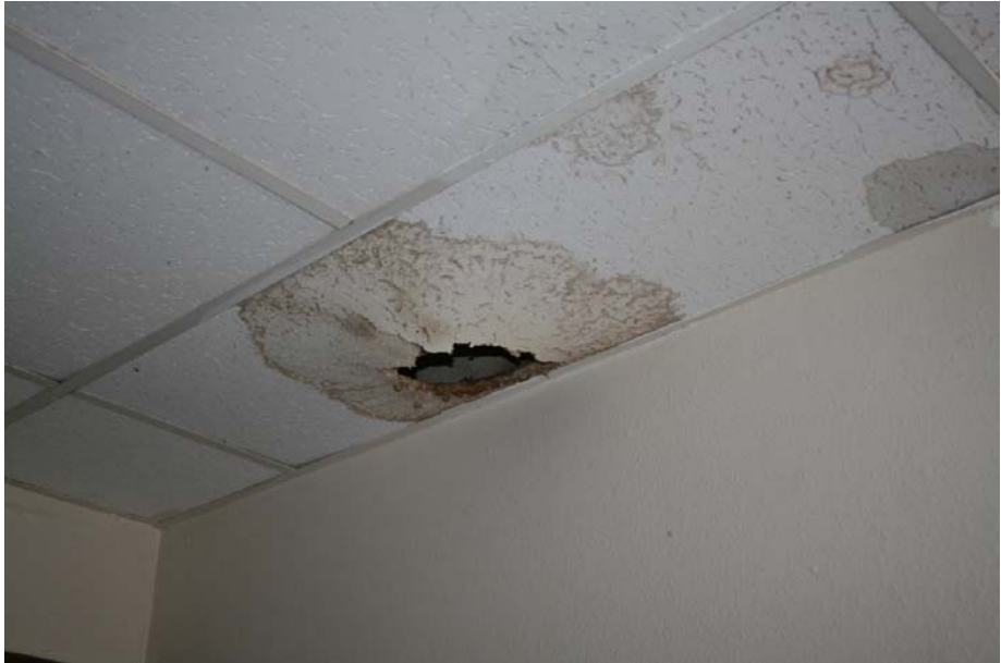
Unit 33: Hole in ceiling; active leak from bathroom above
