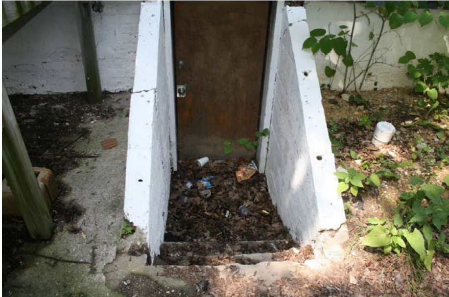
Unit 46: Stairs to basement; no handrail, stairs covered in debris, and dangerous tripping hazard
