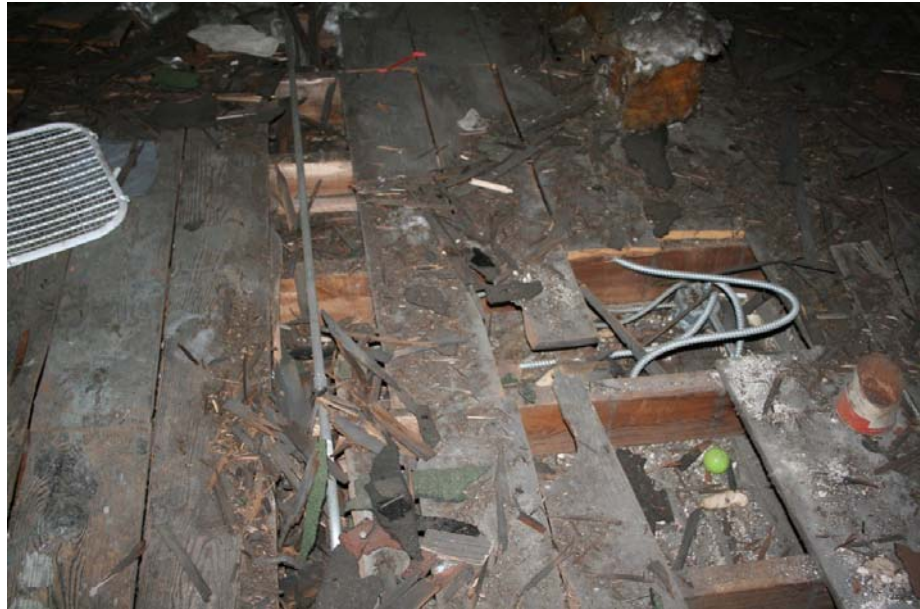
Unit 40: Deteriorated floor in attic used for a bedroom
