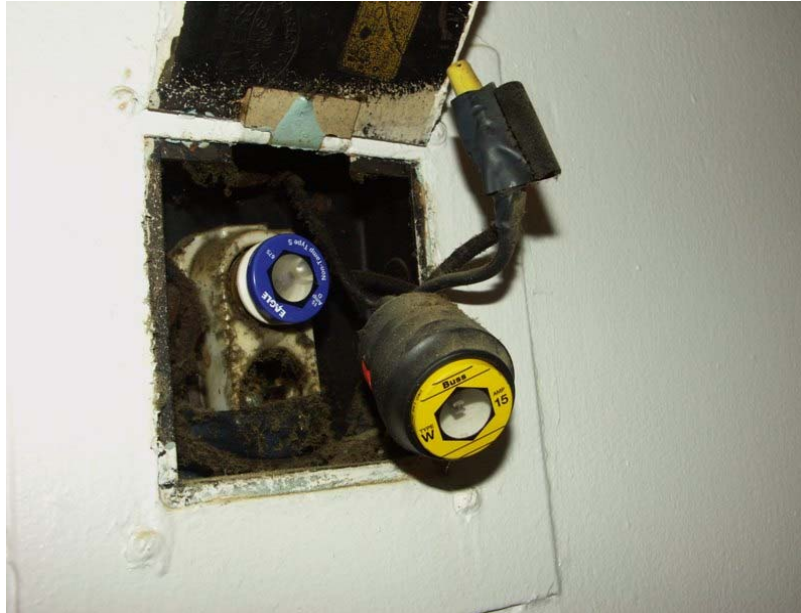
Exposed fuse covered with dirt.
