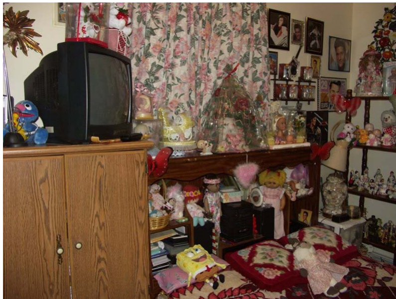
Furniture and personal effects block the window in a bedroom, preventing exit or fire department entry in an emergency.
