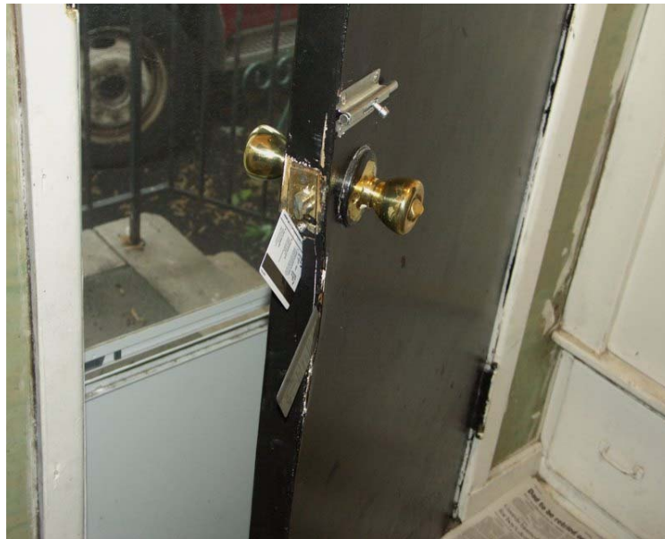
Damaged entry door with significant splits and missing strike pad.
