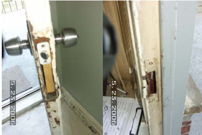
Damaged main entrance door with damaged door frame and strike pad.
