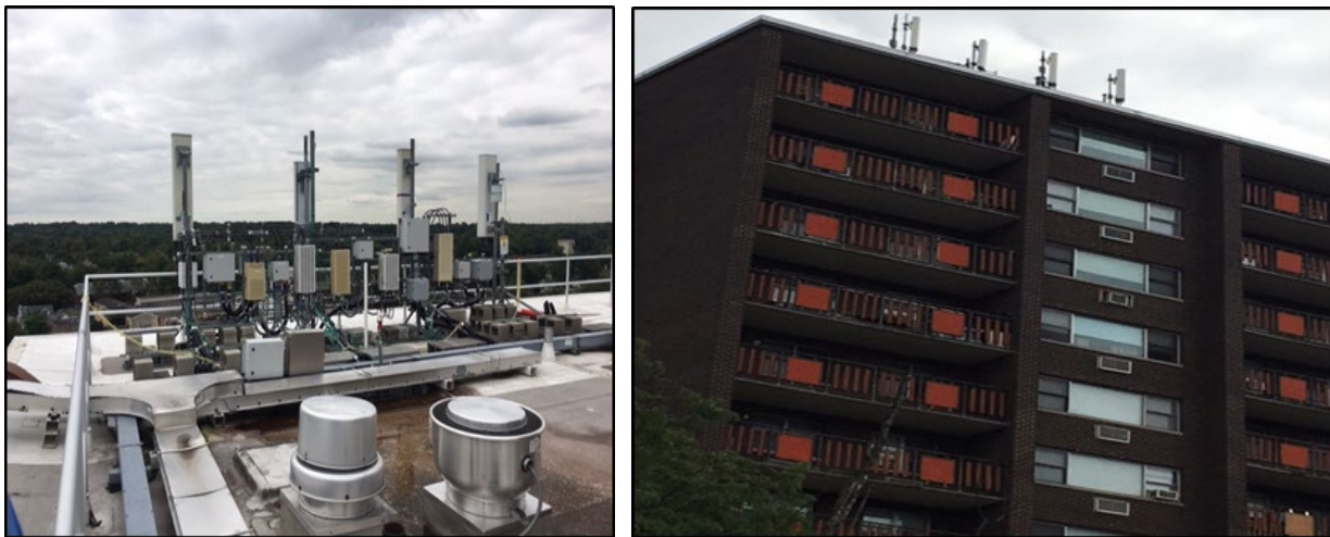
Pictures showing the use of a project rooftop for cell phone towers
