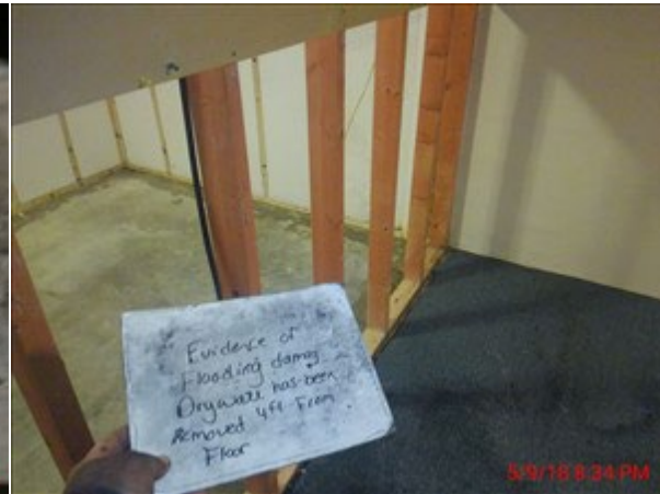
Photo showing inspector's note that there is evidence of flooding damage and that drywall has been removed 4 feet from the floor.
