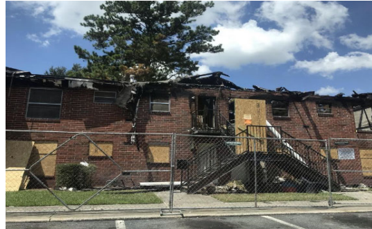
Aftermath of the apartment fire at Calloway Cove caused by a gas leak at the property
