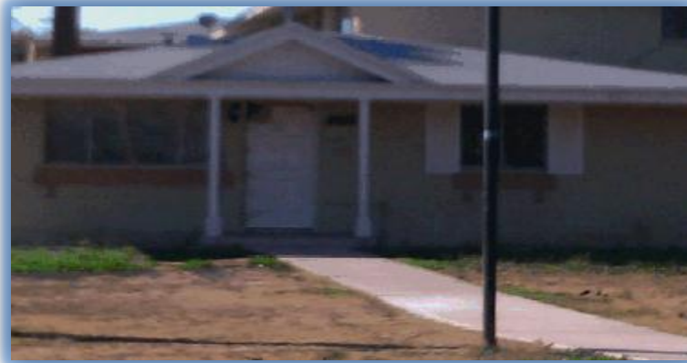
Picture 2: “Block 11” building that needs painting more than seven months after the contractor represented that “paint” was complete and one and a half months after the contractor represented that “Alternate 2 Exterior (sic) Painting” was complete (February 2012)
