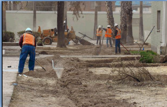
Picture 4: Irrigation system installation more than 4 months after the contractor represented that irrigation was complete (October 2011)
