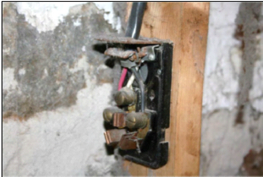
Inspection #46: The 220-volt outlet was missing a cover, exposing the electrical wiring. The Authority did not identify this violation during its October 15, 2013, inspection.
