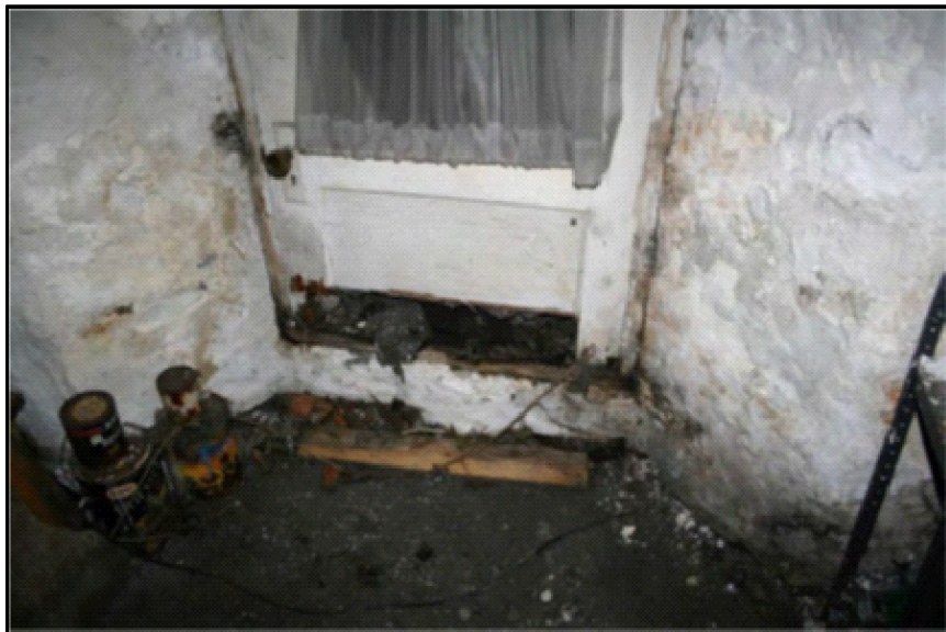
Inspection #59: The basement door was rotted and was missing the bottom section, allowing water and other outside elements to enter the basement. The Authority did not identify this violation during its October 2, 2013, inspection.
