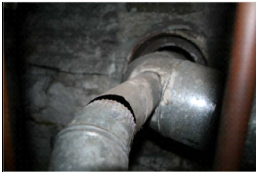
Inspection #24: The furnace and hot water heater flue pipes located in the basement were not sealed, allowing fumes to enter the unit. The Authority did not identify this violation during its August 29, 2013, inspection.
