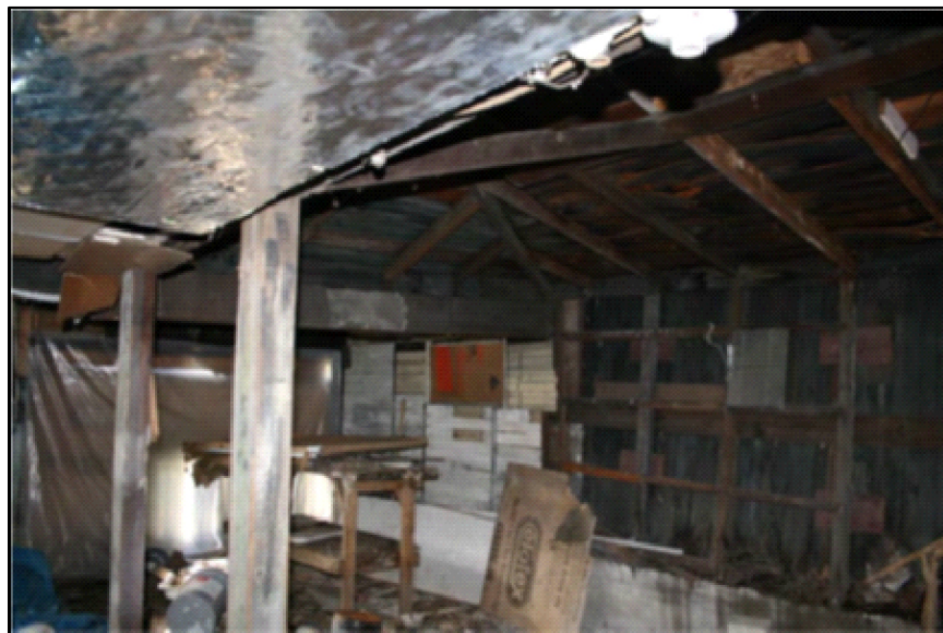
Inspection #57: The unit's garage was not structurally sound. Support beams were used to hold the ceiling in place. Additionally, the side wall was rotted at the bottom, allowing the wall to lean. The unit's kitchen was located above the garage. The Authority did not identify this violation during its October 8, 2013, inspection.
