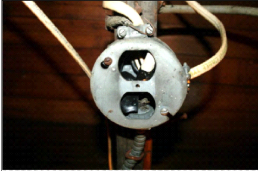
Inspection #67: The junction box located in the basement of the unit had the wrong cover, exposing the electrical contacts inside the box. The Authority did not identify this violation during its September 27, 2013, inspection.
