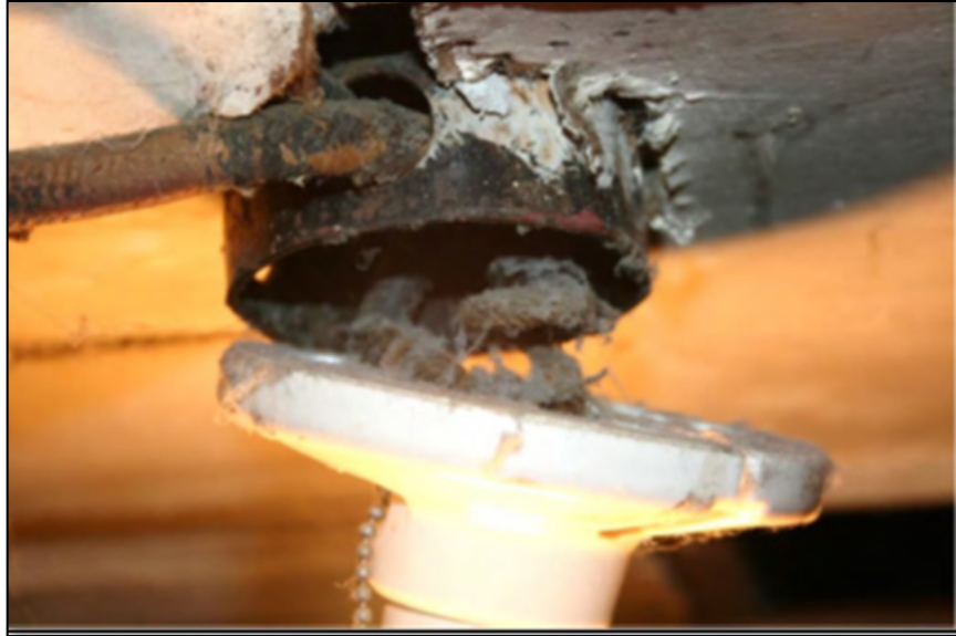
Inspection #46: The ceramic light fixture was not secured to the junction box, and the romex connector was missing. The Authority did not identify this violation during its October 15, 2013, inspection.
