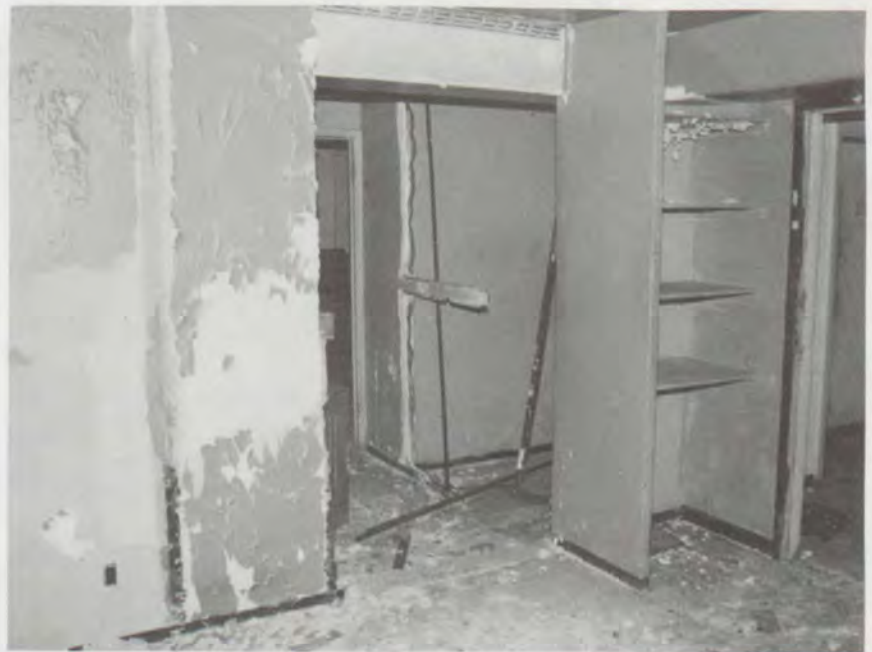
An example of one of the unit's interior was typical of most of the units and depicts the absence of any work performed.
