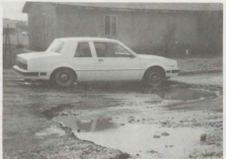
Streets are in need of repair because of lack of maintenance. The maintenance responsibility has not been transferred to the tribe.
