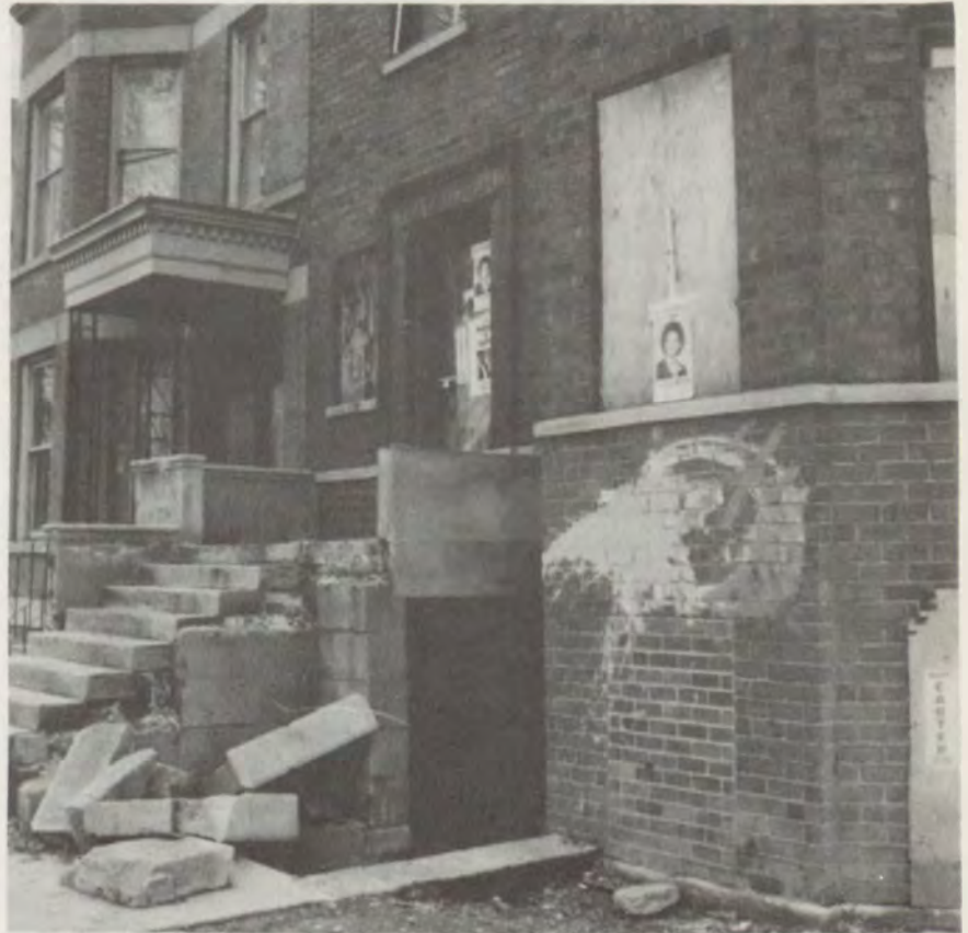
Over $218,000 was already spent for rehabilitation work on this 6-unit structure managed by the CHA. We estimate that it will cost $212,000 more to complete rehabilitation than to build a new structure.
