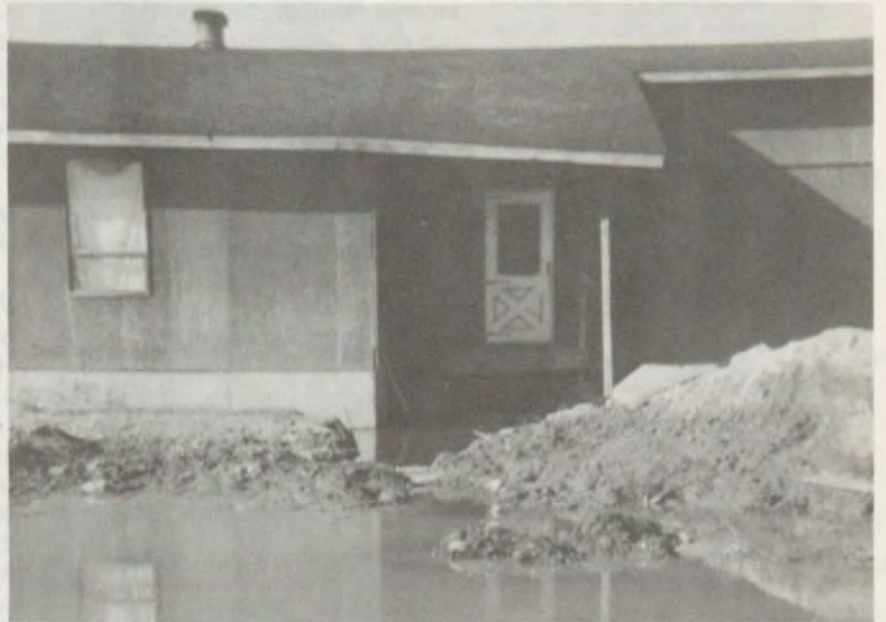
Water from an unknown source has caused structural damage to this house.
