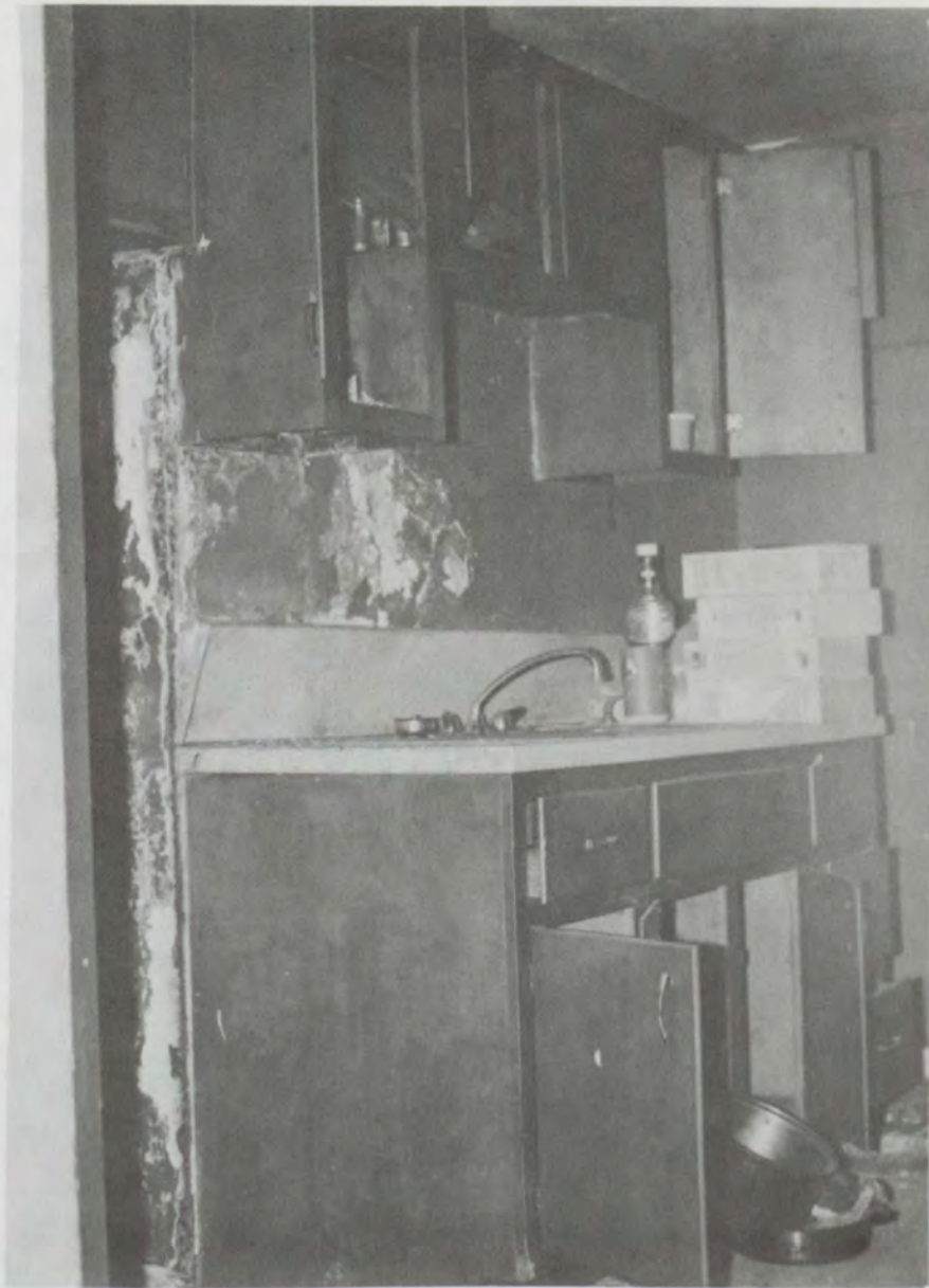
Example of CMHA unit requiring extensive repairs before occupancy.
