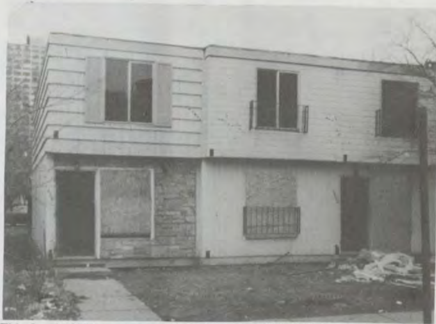
This 8-unit CHA structure still requires over $280,000 for repairs. Since the buildings are not structurally sound, we believe it may not be cost efficient to rehabilitate the structure.
