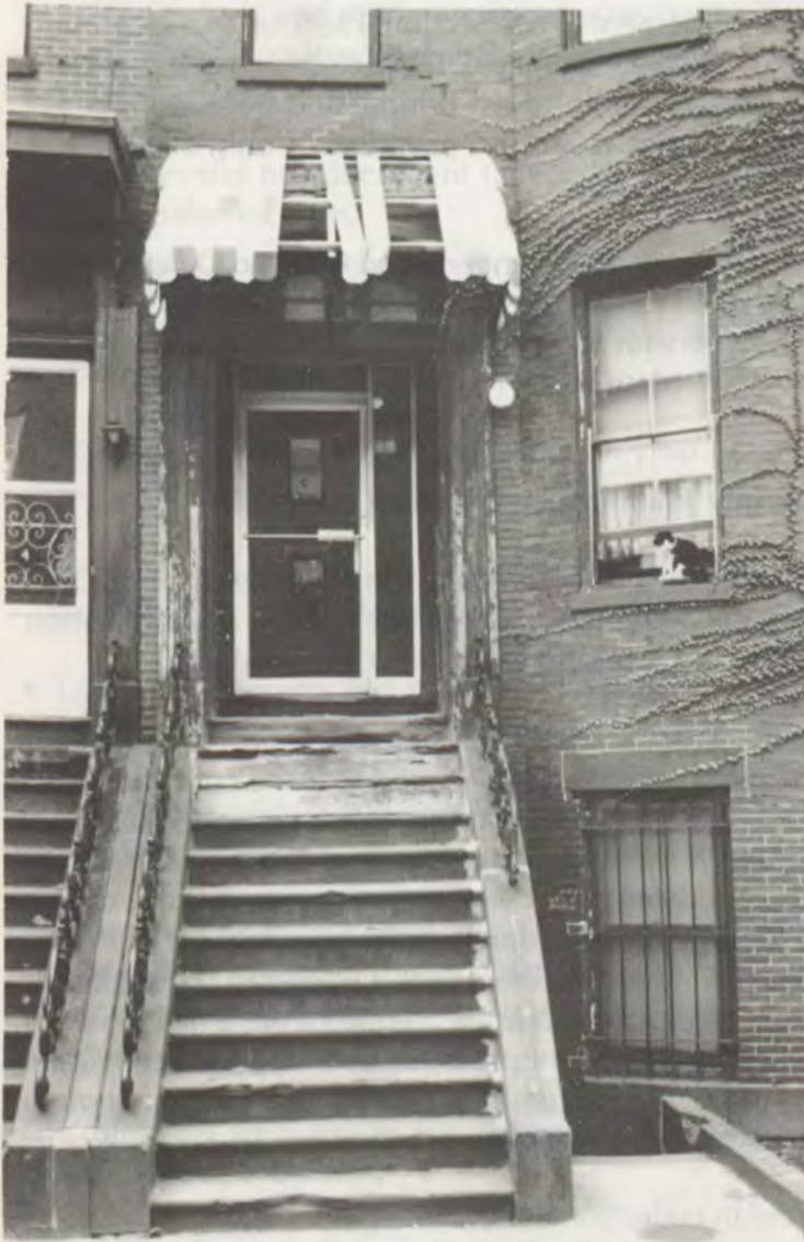
Entrance steps are deteriorated, and rail and sections of canopy are partially missing.
