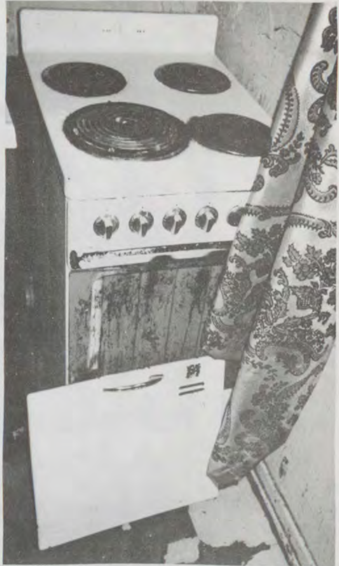
Inoperable stove. Detroit tenant said the stove "blew up" over a year ago and she has yet to receive a requested replacement. Note that the stove is adjacent to a window with curtains and represents a fire hazard.
