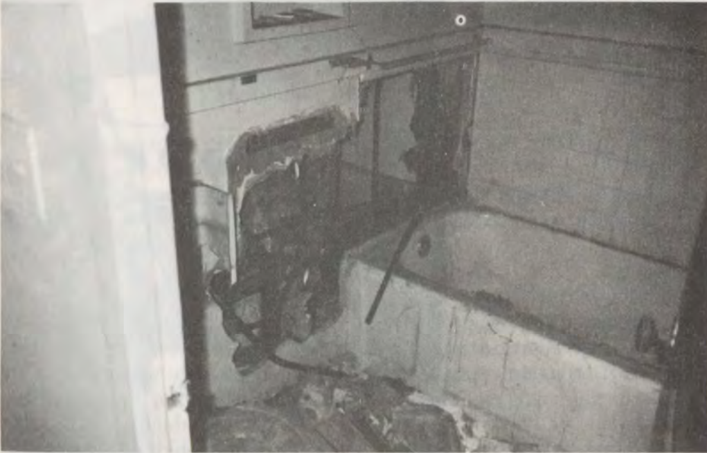
This unoccupied unit managed by the Detroit PHA shows severe damage. The photograph is representative of many unit interiors.
