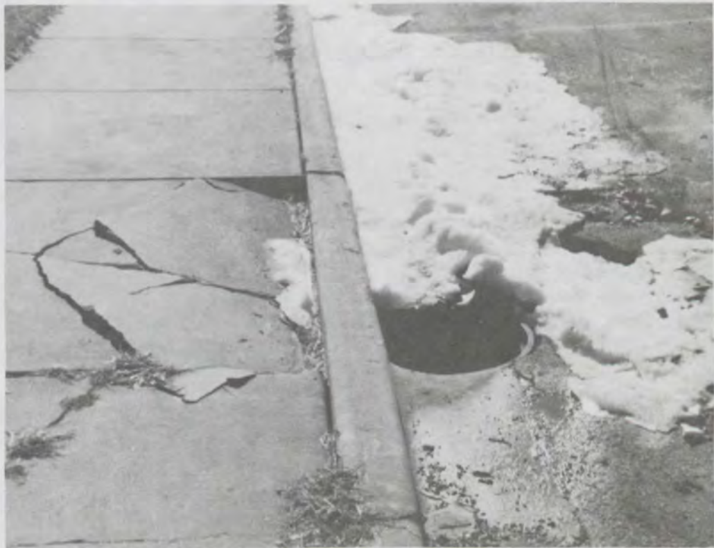
Deteriorated and unsafe walkway and driveway (note the open manhole) near an occupied building at Concordia Park in Detroit.
