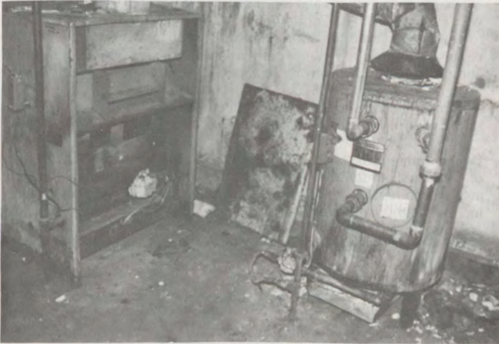
Corroded and deteriorated heating unit in an occupied building.
