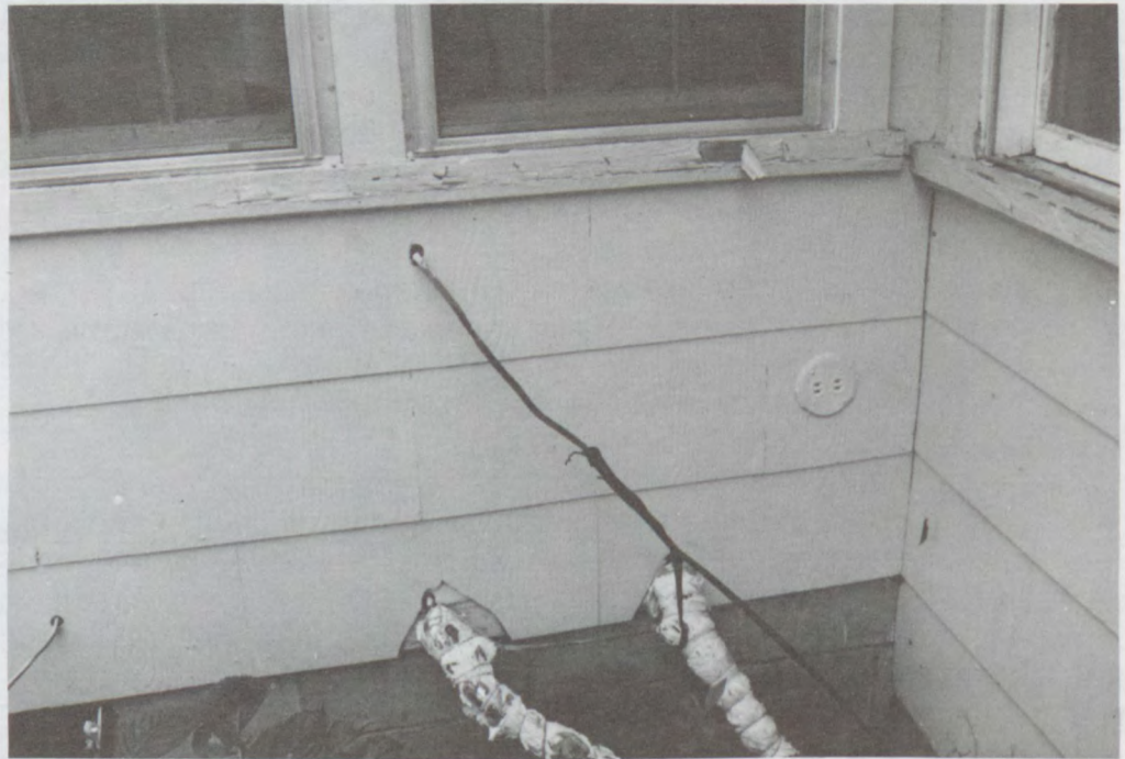
Peeling exterior paint and hazardous electrical wiring at SCSHA project.
