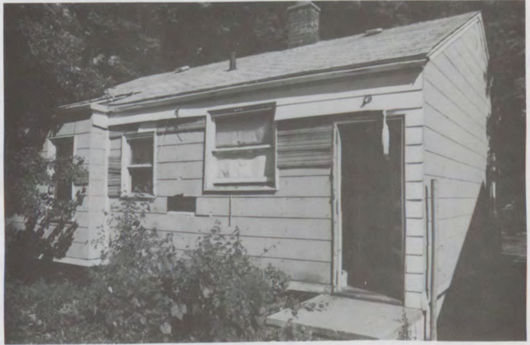
Both photographs show vacant, open, vandalized properties in Detroit, Michigan. Mortgages on both properties had been placed in an "inactive" inventory and no actions were being taken by the Detroit Office.
