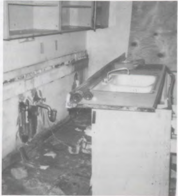
Severely damaged kitchen - Parkgate Apartments Kansas City, MO
