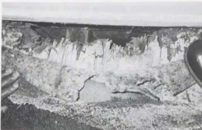
Rotted floor - French Village Apartments, Kansas City, MO
