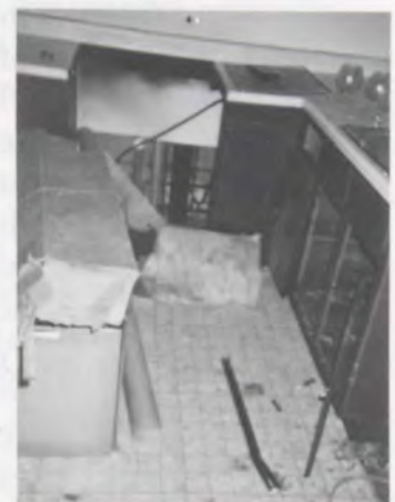
Intensified deterioration caused by lack of routine maintenance - French Village Apartments, Kansas City, MO
