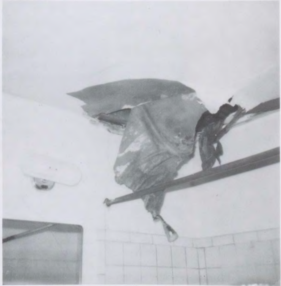
Rotted bathroom ceiling - Parkgate Apartments, Kansas City, MO
