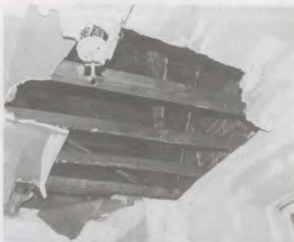
Bedroom ceiling that has caved in due to plumbing leaks from upper units.
