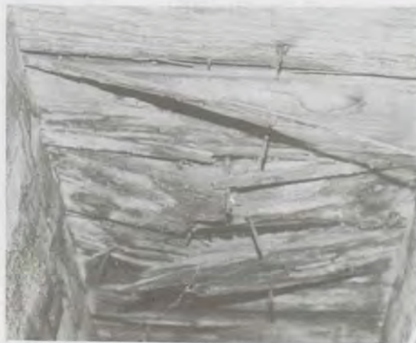
Rotted kitchen subfloor at uninhabitable PHA unit.
