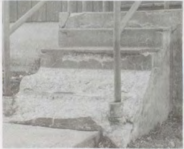
Hazardous entry steps.
