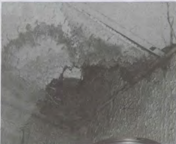
Severely deteriorated wall and ceiling at unit with 11 Housing Quality Standards violations (HUD standards of decent, safe and sanitary housing which all units must meet before rental by program participants).
