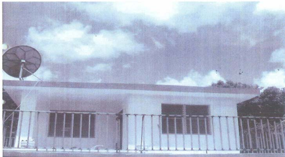
Figure 7: Case Number 2002-099- After Rehab
