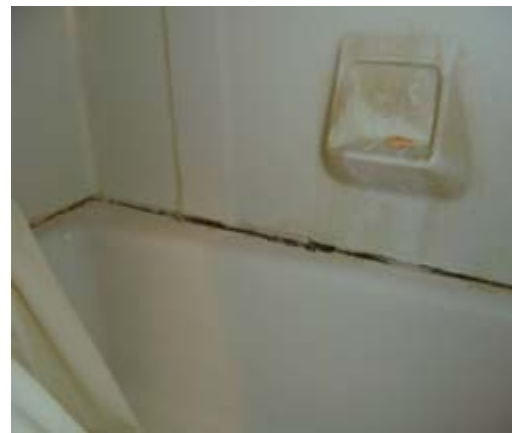
Mold around a bathtub
