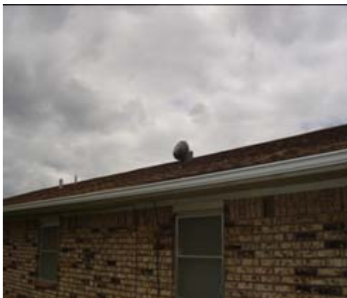
Broken roof turbine exposing the unit to water and small animals
