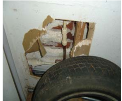
Hole in a garage wall that exposed pipes
