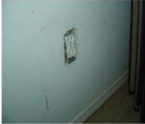
Missing electrical outlet cover plate
