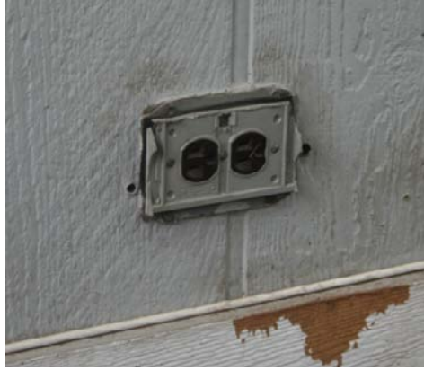
Exposed electrical outlet without safety cover
