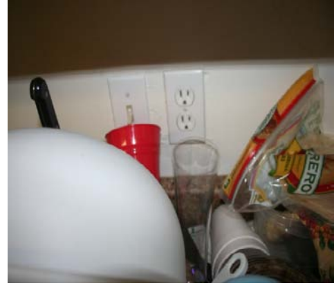
Missing GFCI outlet in updated kitchen
