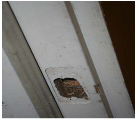
Missing door striker to rear entrance
