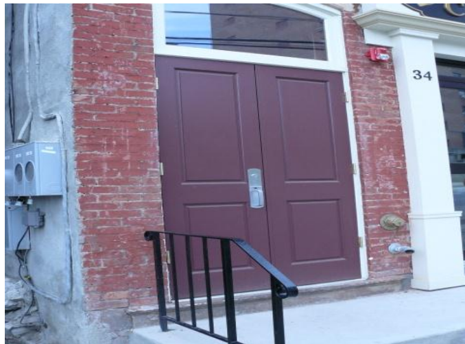
This photo shows that only one decorative railing was installed.
