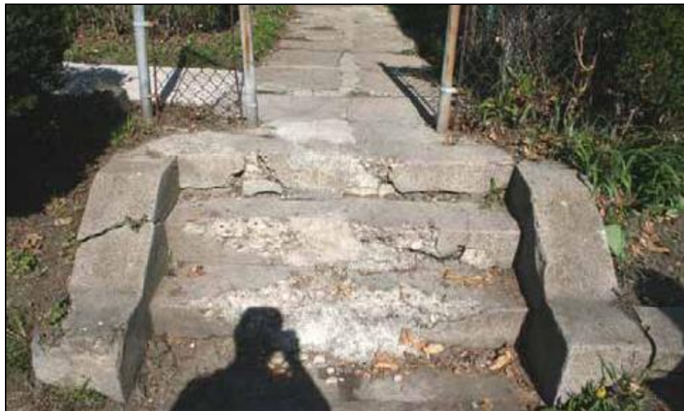
Inspection #42: The concrete steps are chipped and broken. The steps need resurfacing and a handrail. This violation was not identified during the Authority's October 31, 2007, inspection.
