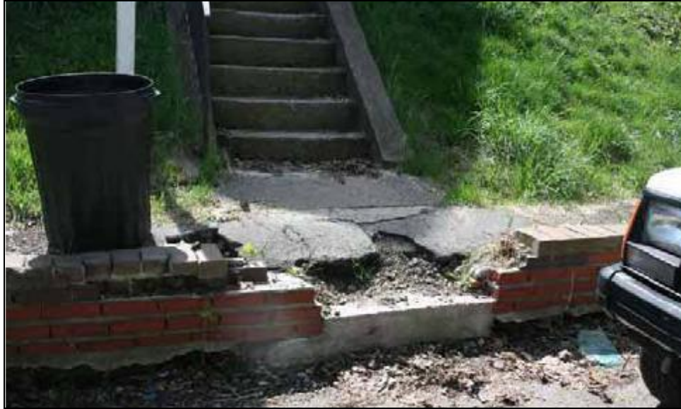
Inspection #8: The step from the street to the walk, as well as the sidewalk, needs to be repaired. This violation was not identified during the Authority's October 10, 2007, inspection.
