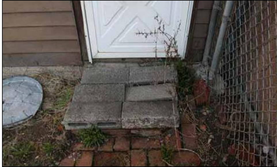
Inspection #26: The landing at the exit from the rear door is uneven. This violation was not identified during the Authority's September 27, 2007, inspection.
