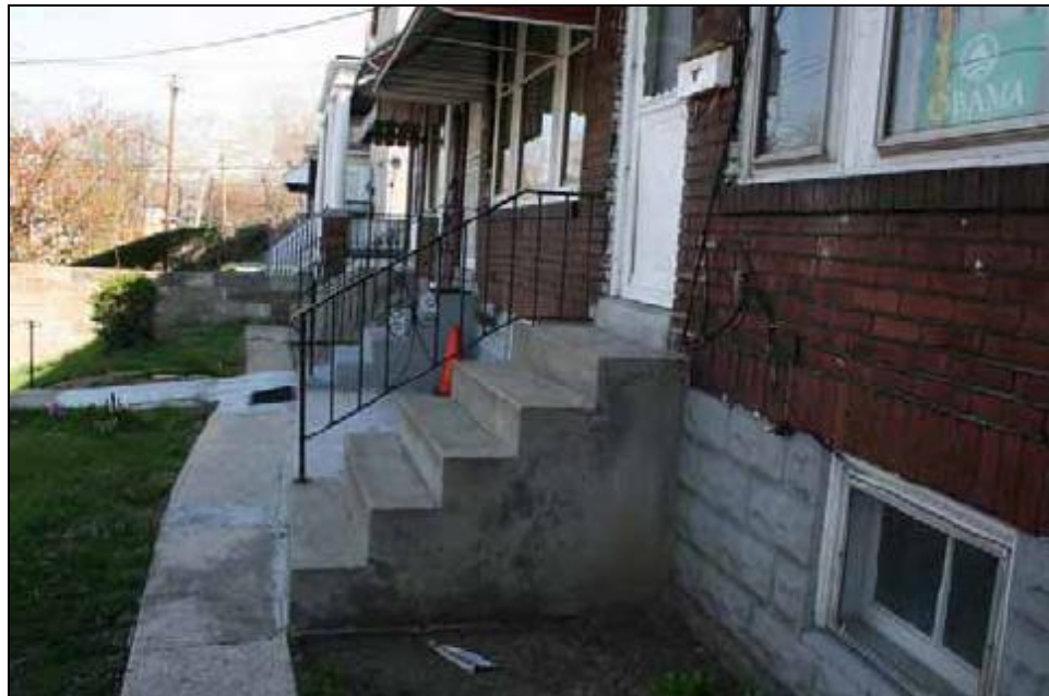
Inspection #36: A handrail needs to be installed on the right-hand side of the steps or
