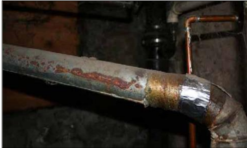
Inspection #8: The hot water heater flue is rusted and needs to be replaced. This violation was not identified during the Authority's October 10, 2007, inspection.
