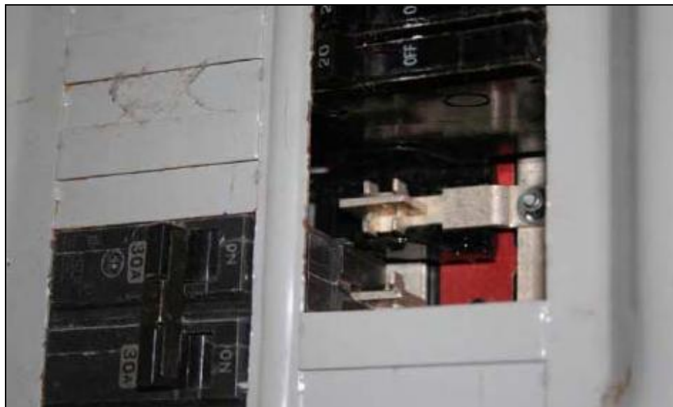
Inspection #11: Knockout plugs are missing from the breaker box. This violation was not identified during the Authority's November 19, 2007, inspection.
