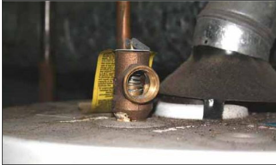
Inspection #38: The drain tube is missing from the pressure relief valve. This violation was not identified during the Authority's November 19, 2007, inspection.
