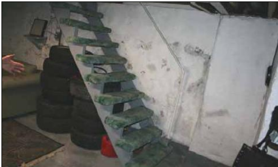
Inspection #6: A handrail is missing on the right-hand side of the basement stairs. This violation was not identified during the Authority's November 14, 2007, inspection.
