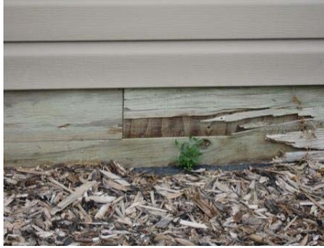
Exterior wood not pressure treated
