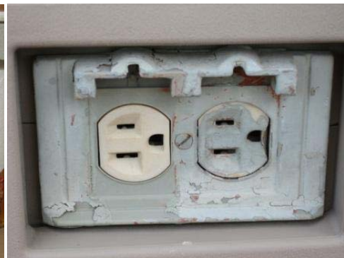
Exterior outlet no GFI or cover
