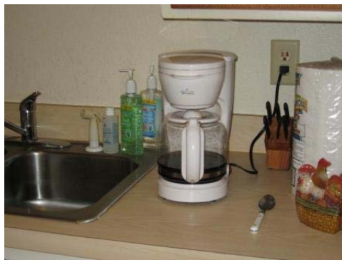
Kitchen outlet no GFI
