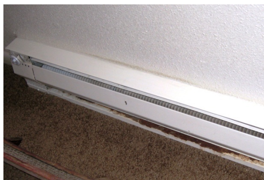
Rusted baseboard heater
