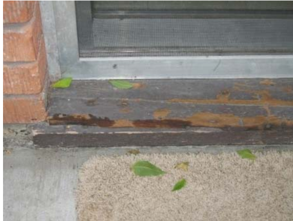
Rotten wood under sliding glass door threshold
