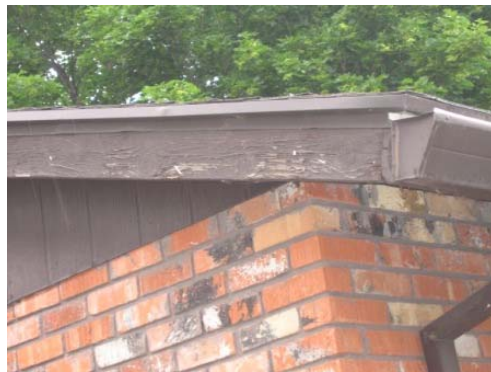
Trim paint flaking
