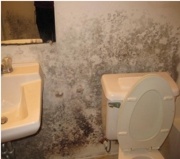
Picture 3: Vacant unit – mold in walls
