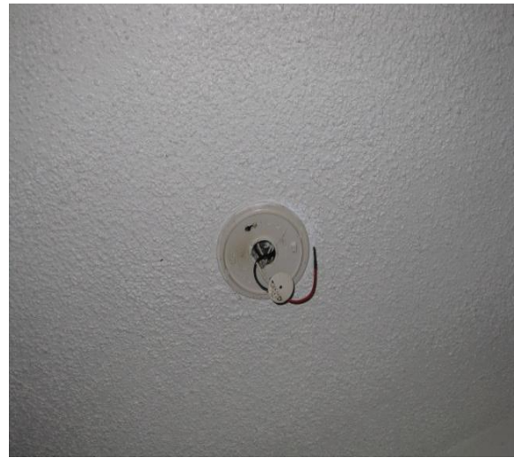
Picture 6: Occupied unit – missing smoke detector
