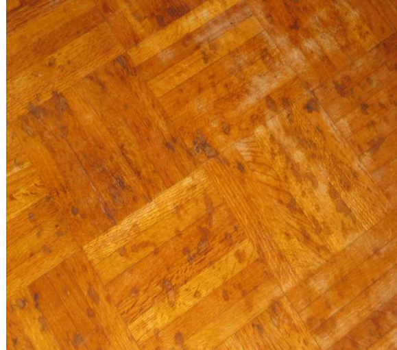
Picture 8: Occupied unit – moldy floors
