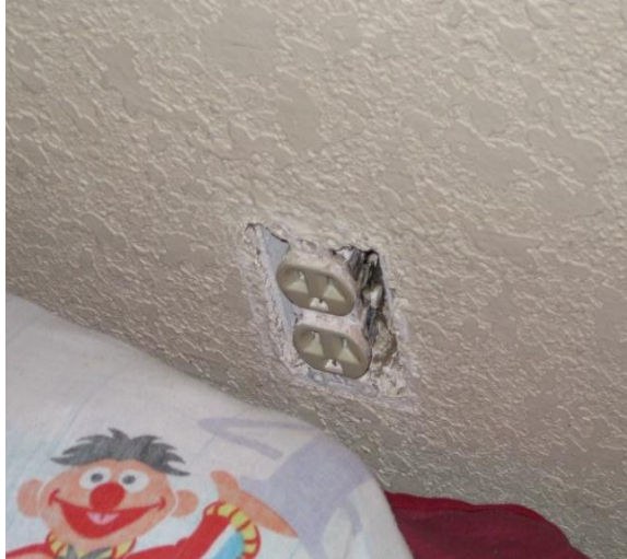
Picture 7: Occupied unit – missing outlet cover
