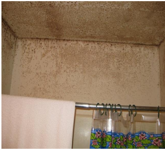
Picture 5: Occupied unit – mold on walls and ceiling
